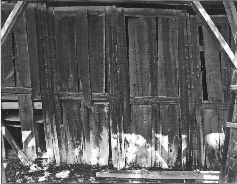
Severe shrinkage of the wall panels had rendered the sides no longer tight and well fitted. Nails were required to hold the structure together.
